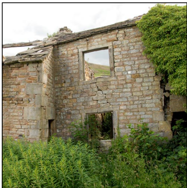
Figure 7. Distortion by ground movement of the old Callow Bank Farm, showing in the fracture through the stonework between the two window openings.
